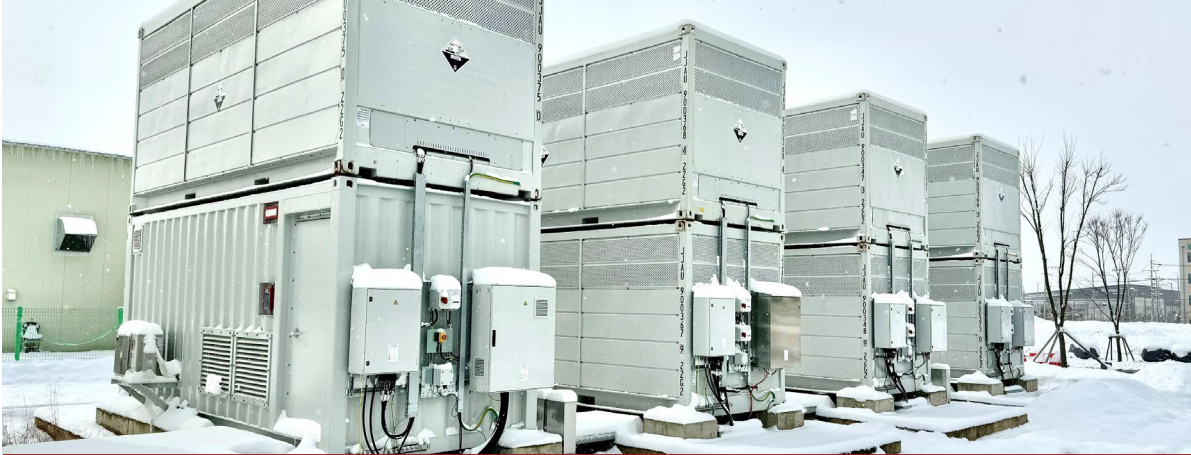
HIGH THROUGHPUT DEMONSTRATOR / KEPCO Grid Services 1.5 MWh
